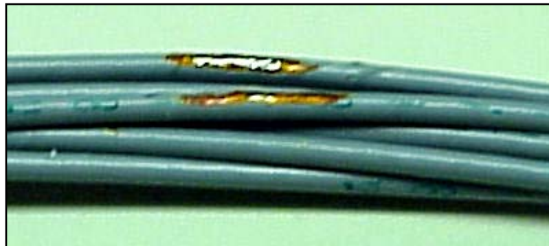
Damaged wires prior prone to arc over
